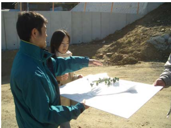
[Photo 1] Students designed Awaji City's first park for urban blocks. Shown here are students carefully examining the model at the construction site.
